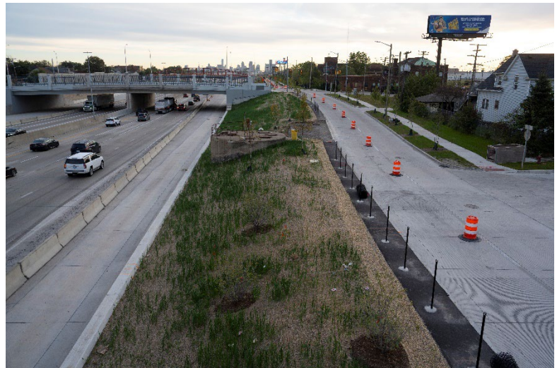
I-75 Service Drive local road improvement work between Wheelock Street and Green Street.
