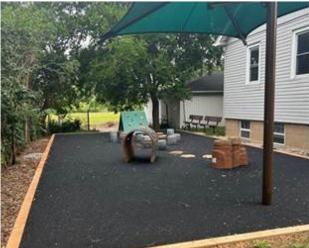
Work on the accessible playground at the Summit Centre for Preschool Children with Autism progressed over the summer months.
