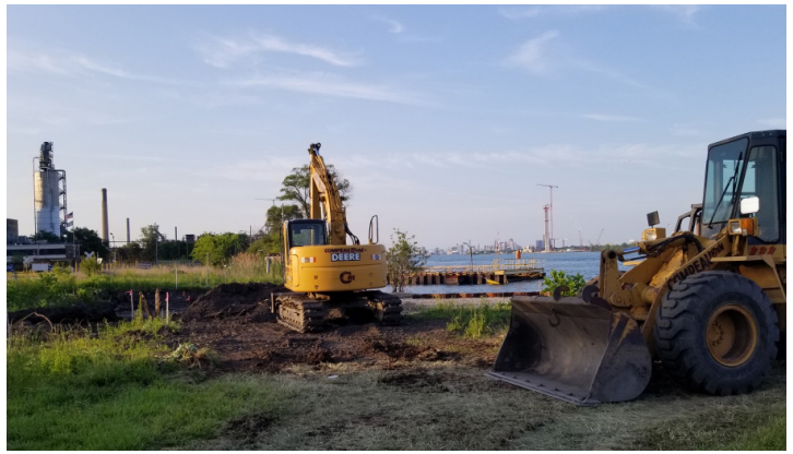
Site grading took place in the summer to prepare for construction of the observation area in River Rouge.
